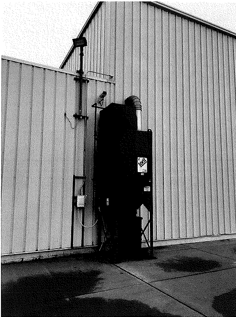
Image 4(12) : Exempt Torit controls equipment in the Tooling Room
