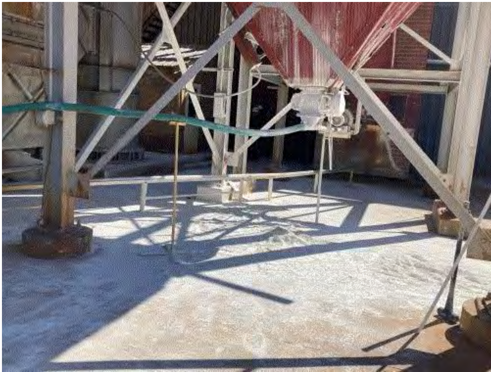
Image 2(Lime) : Lime noted on ground near baghouse. This is the result of baghouse changeout.
