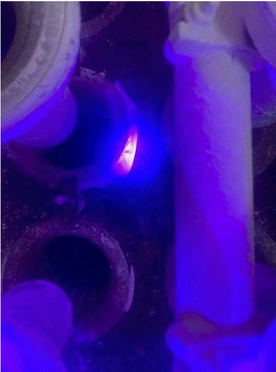
Image 7(Trace Baghouse) : UV Trace Light indicates leaks around the seal of a bag contained within KILN01's baghouse.
