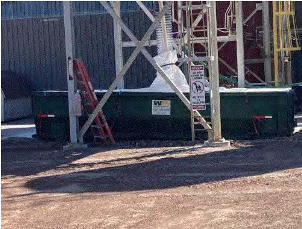
Image 4(Waste Lime Bin) : System implemented to collect waste lime from storage silo.
