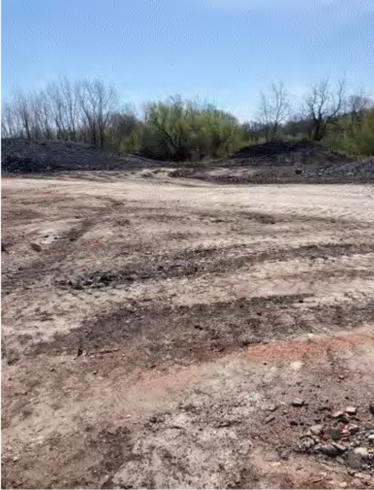
Image 6(Haul controlled) : Photo taken by Michigan Brick on 4/19/23. Photo used to demonstrate water was applied to the haul road to minimize fugitive dust from truck traffic.
