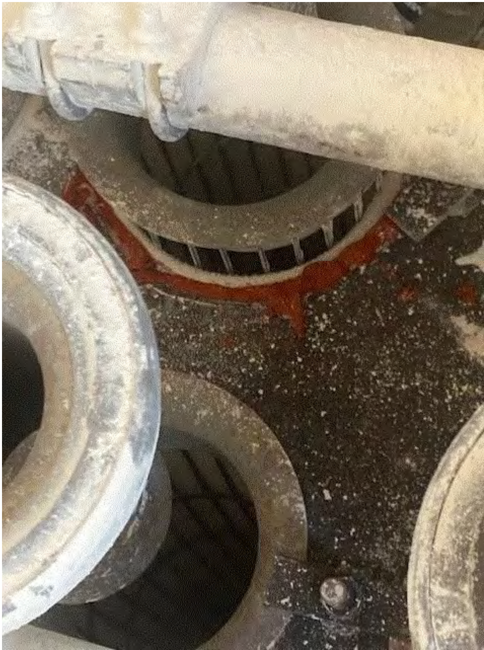
Image 9(Caulked Bag) : Photo Credit: Michigan Brick. Photo shows caulk has been applied at seal of bag cage.
