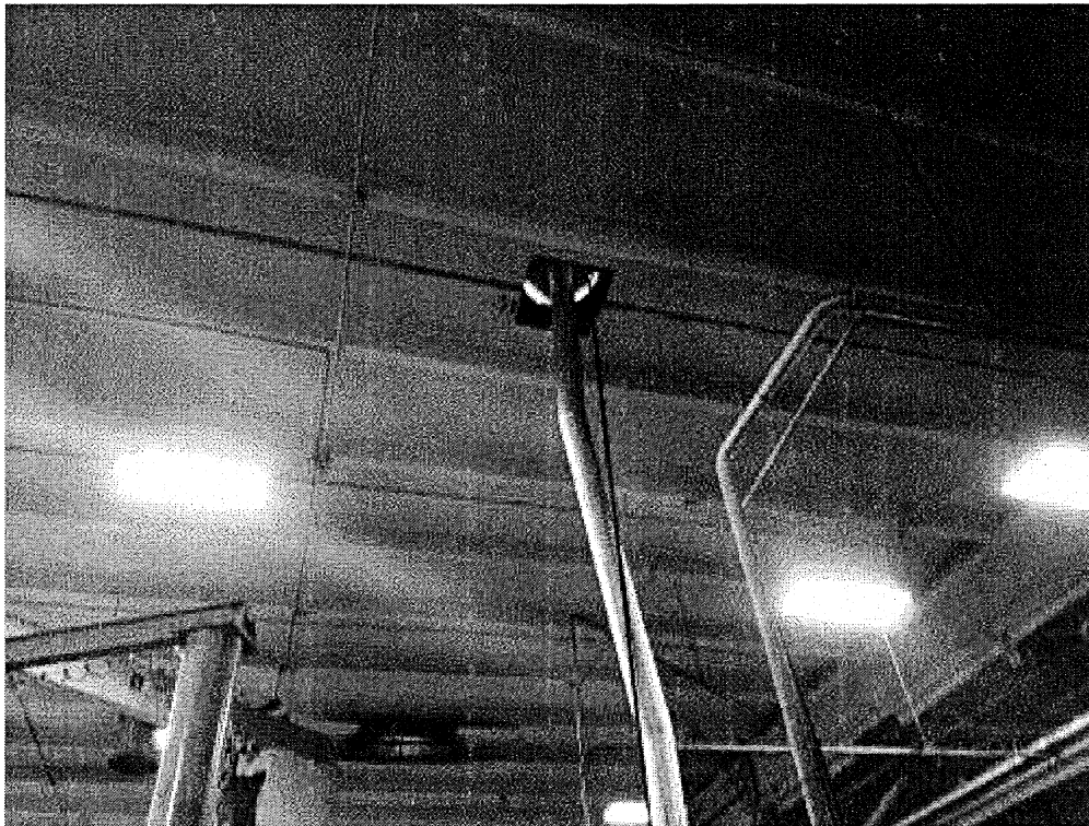
Image 16(Furnace stack) : Furnace stack
