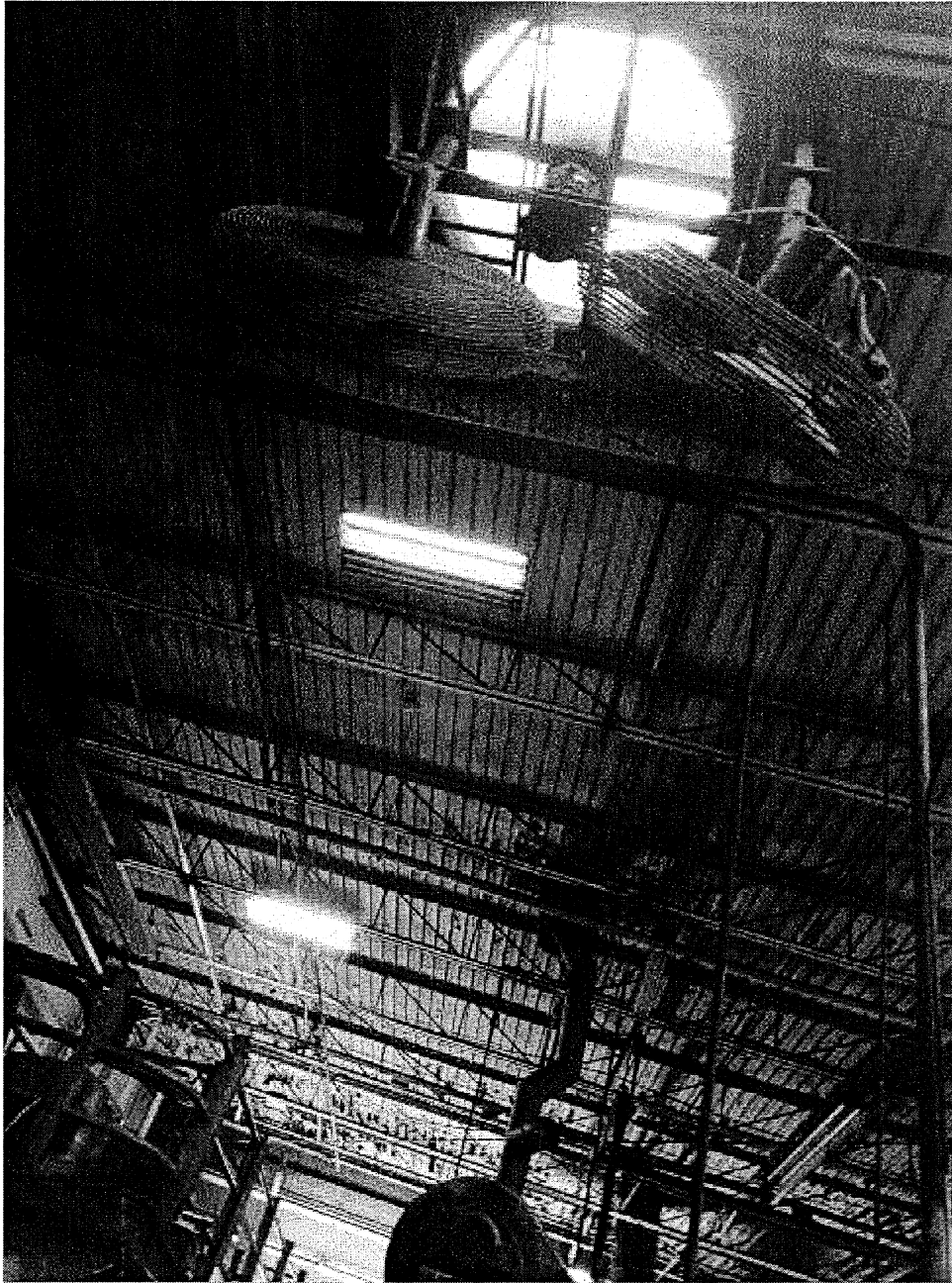
Image 19(Ceiling fan) : Ceiling fan above furnance
